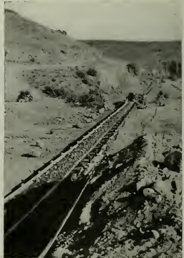
Moving material at average rate of 147 yards per hour, 2600-foot conveyor transports 90,000 yards to upstream portion of dam.
